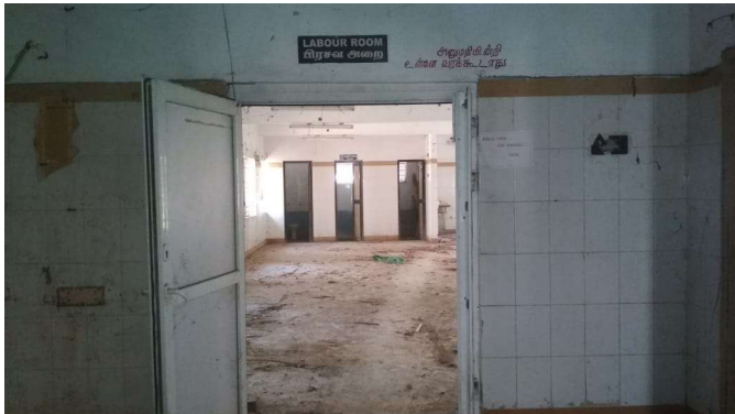
One of the halls in the building allocated to Soulfree for the construction of our SCI Rehab Centre
